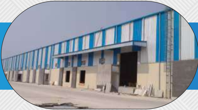
Project – Oriclean Pvt Ltd, Cuttak Odisha, 200000 Sq Feet Project Type – Warehouse for HUL
