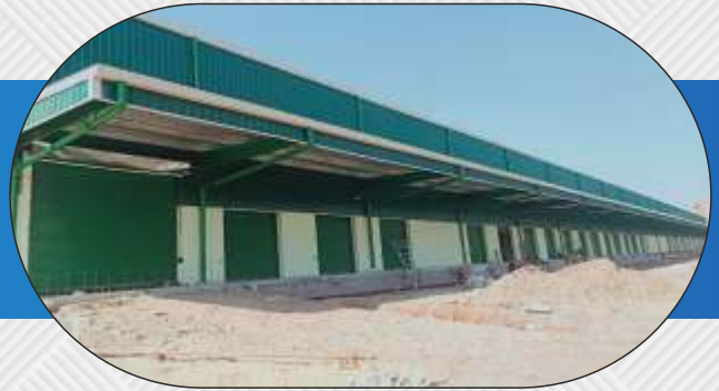
Project – Shiv Pujan Marchents LLP, Bhuvneshwar Odisha 125000 Sq Feet Project Type – Warehouse for Safe Express
